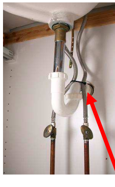
Identify cold water line
